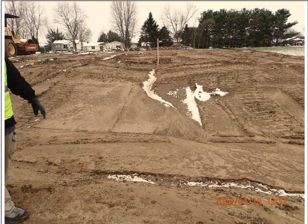
2026.03.18 // Crossing Subdivision, Phase 2 & 3 – Looking west at the north end of Lots 51 A & B and 52 A & B. The fill is encroaching into the drainage swale.
