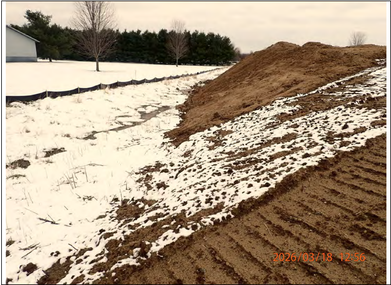
2026.03.18 // Crossing Subdivision, Phase 2 & 3 – Looking northeast at the north end of Lots 55 A & B. The fill is encroaching into the drainage swale.
