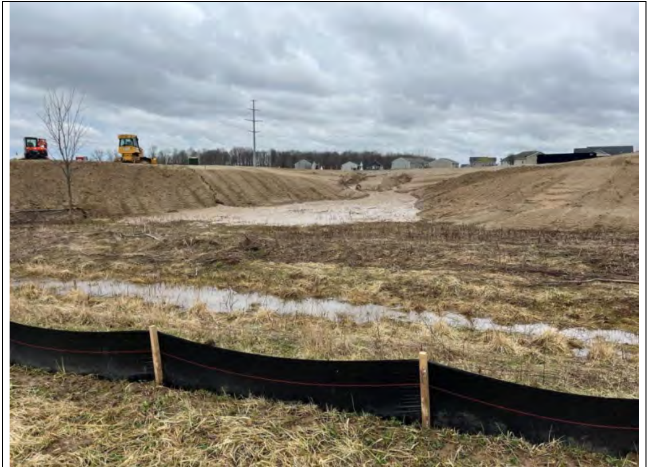
2026.03.13 // Crossing Subdivision, Phase 2 & 3 – Looking southeast at Lots 52 B and 54 B. Significant erosion was observed fanning out into the development lot
