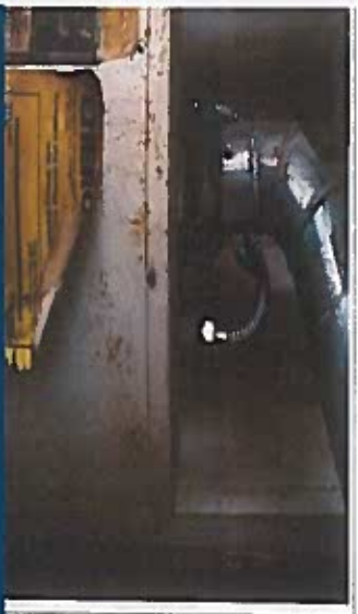
Inoperable water heater
