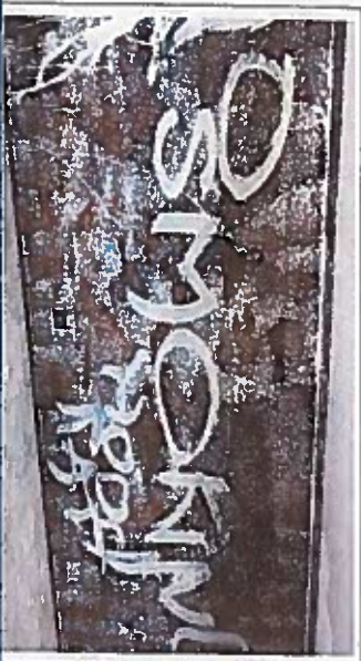
Graffiti & unauthorized access
