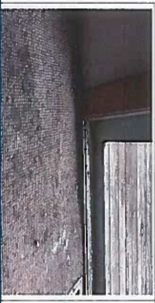
Worn & deteriorated carpet
