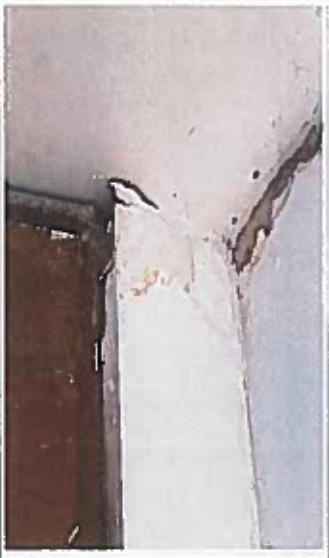
Ceiling separation & water damage
