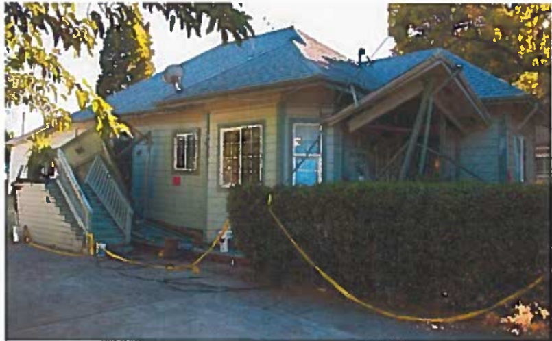
Figure 27: Structural Earthquake Damage
