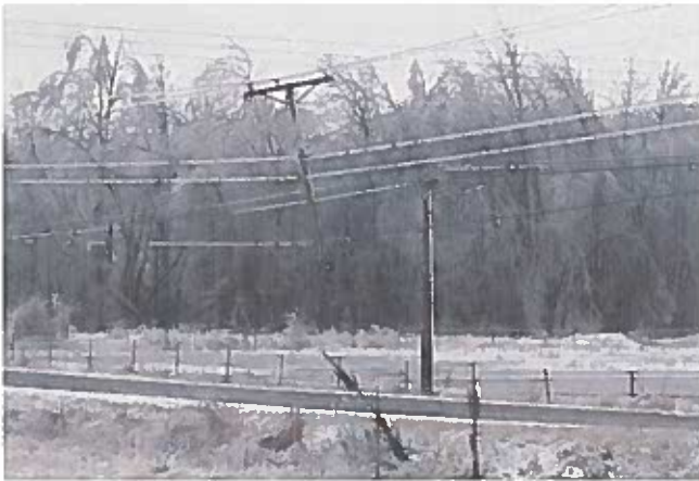
Figure 49 Ice Covered Powerlines
