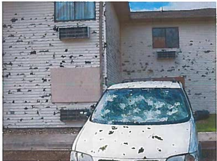
Figure 42 Damage to Vehicle and Structure Caused by Hail
