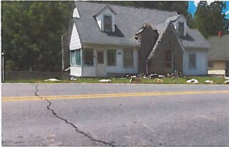
Figure 26: Minor Earthquake Damage
