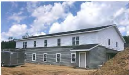
ABOVE: The first of four buildings currently being constructed at Lakeview Drive.
